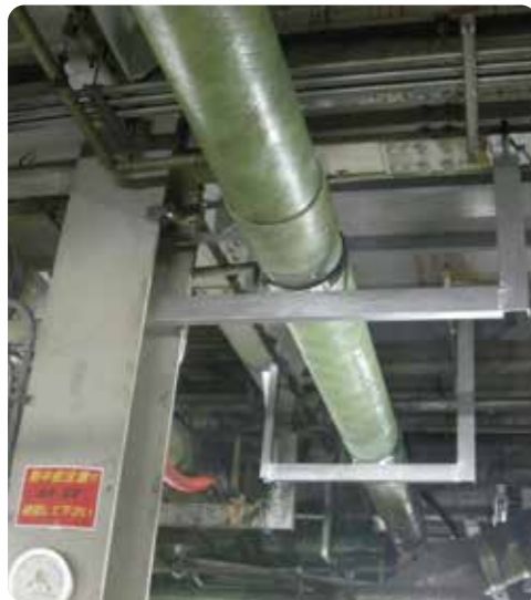
Garbage treatment facility : acid water piping
