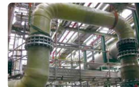
Chemical factory : chemical liquid piping
