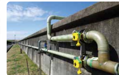
Water purification plant : chemical liquid piping
