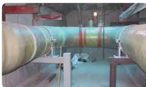
Power plant : seawater piping
