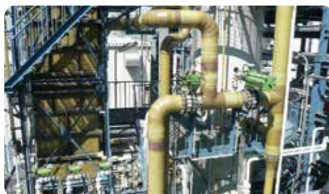
Thermal power plant : duct piping
