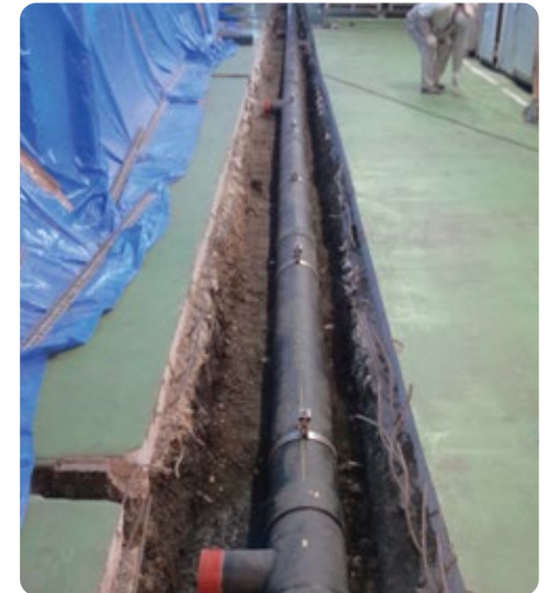
Food factory : drain pipe
