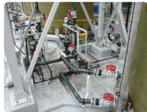
Steelworks : hydrochloric acid equipment, chemical liquid piping
