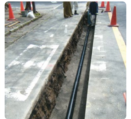
Hot Spring Facility : hot water pipe (with heat insulation)
