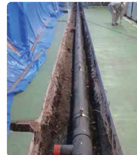
Food factory : drain pipe
