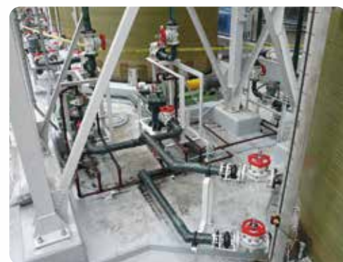
Steelworks : hydrochloric acid equipment, chemical liquid piping
