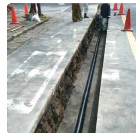
Hot Spring Facility : hot water pipe (with heat insulation)
