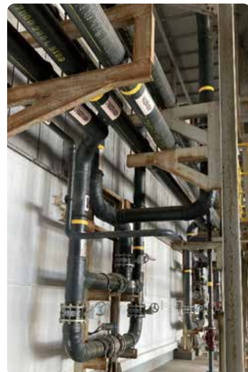
Garbage disposal plant : piping around the smoke washer
