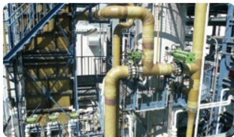
Thermal power plant : duct piping
