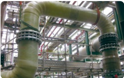
Chemical factory : chemical liquid piping
