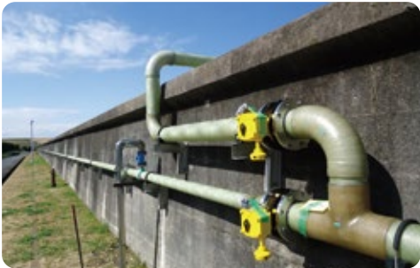
Water purification plant : chemical liquid piping
