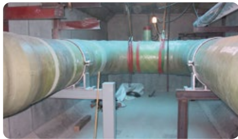
Power plant : seawater piping
