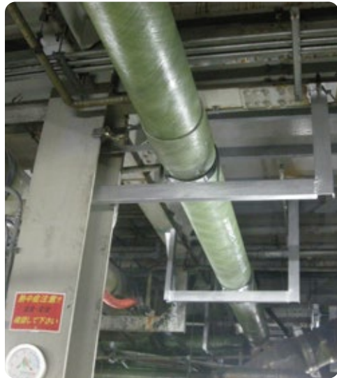
Garbage treatment facility : acid water piping
